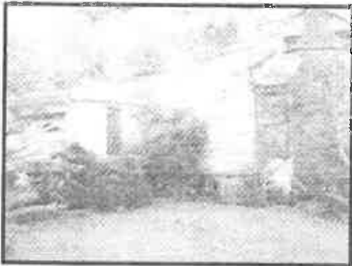
Overgrown Shrubberty Side
